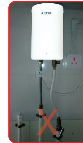
Do not use CPVC Pipes.
