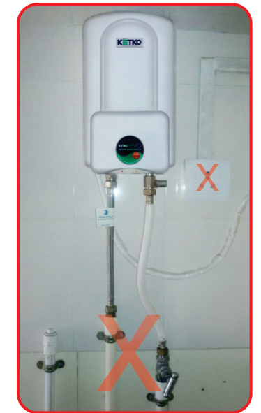
Do not use CPVC Pipes.
